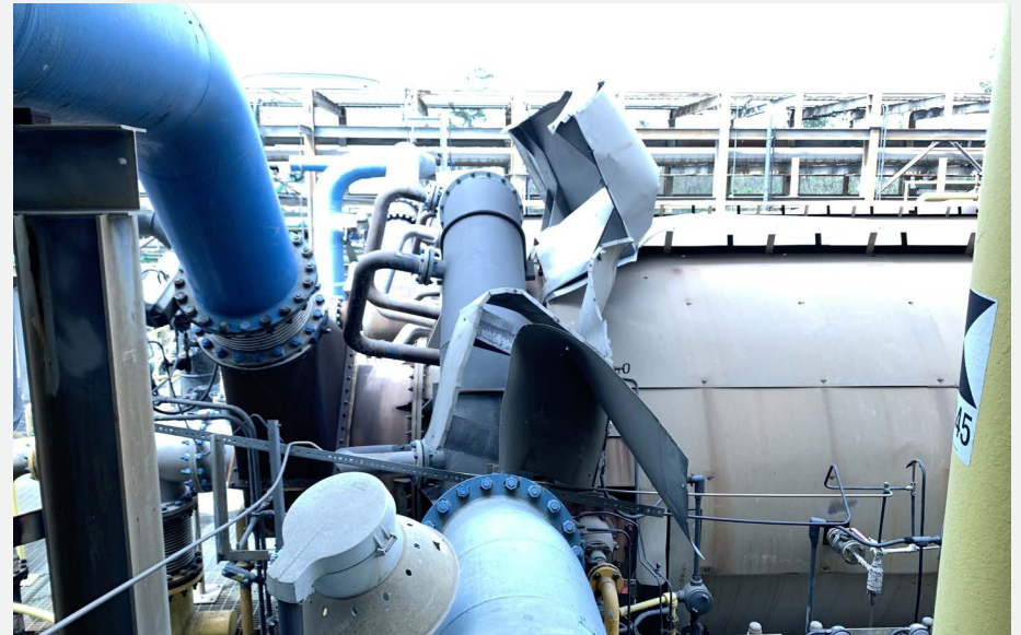
Damaged production equipment.
