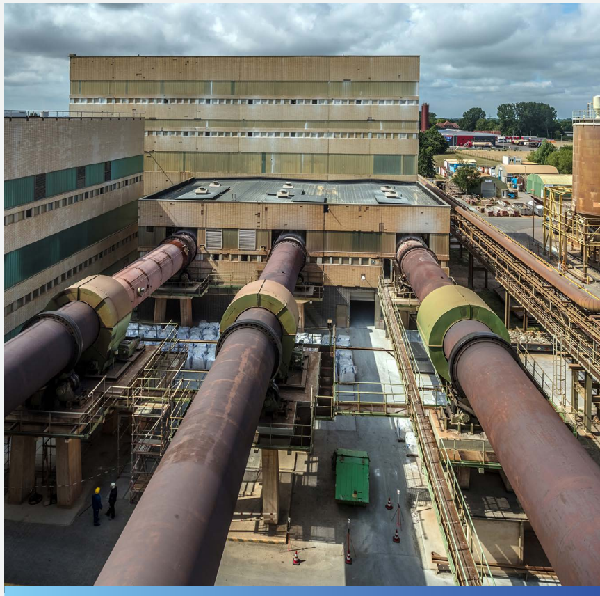
Calciners (rotary kilns) in Nordenham, Germany.
