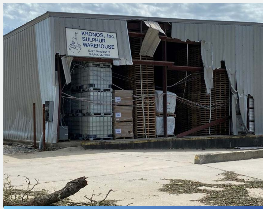
Damage to Louisiana slurry plant and warehouse.
