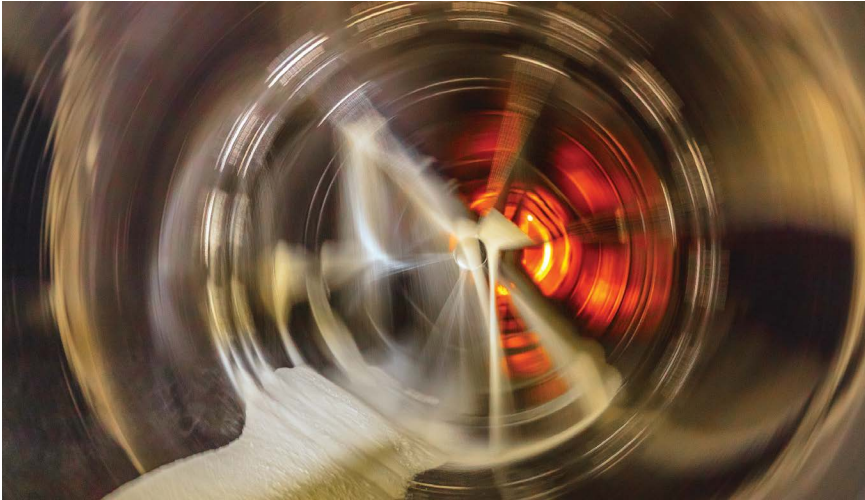
Product cooling drum in Leverkusen, Germany.
