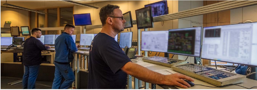
Process control room in Leverkusen, Germany.
