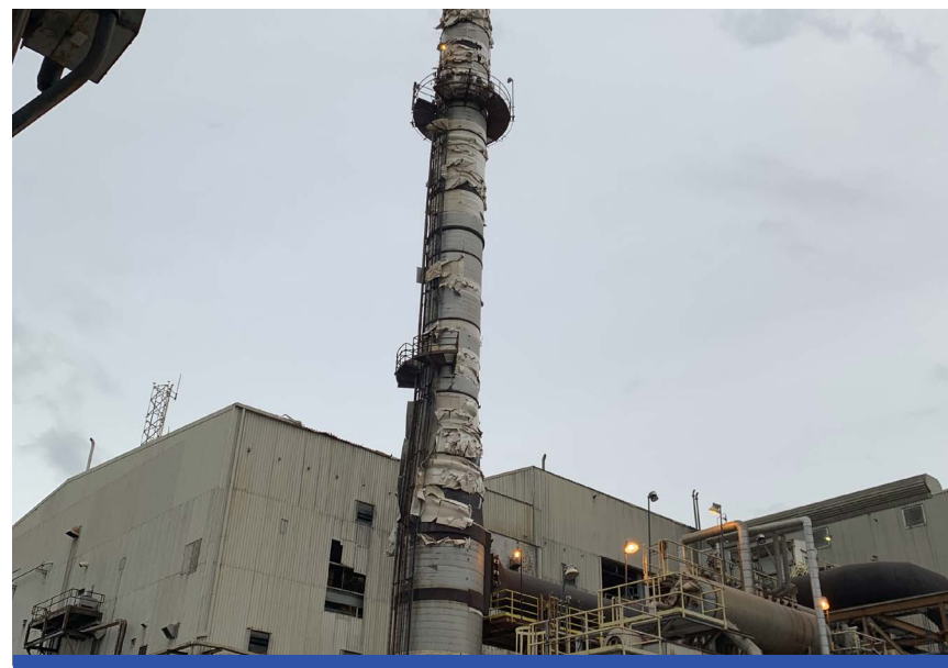
Damage at LPC from Hurricane Laura.
