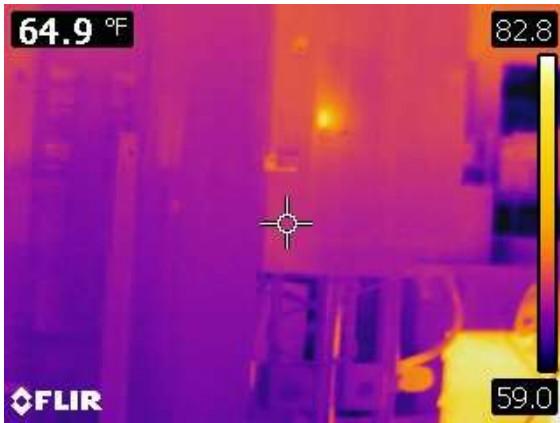
The bright breaker is more loaded than the others, but the 82F is not a concern. If breakers are above 120F, they should be investigated further.
