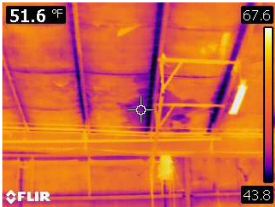
The darkness in the underside of the roof shows a wet spot and could point to roof insulation issues. These issues were seen in ██████████
