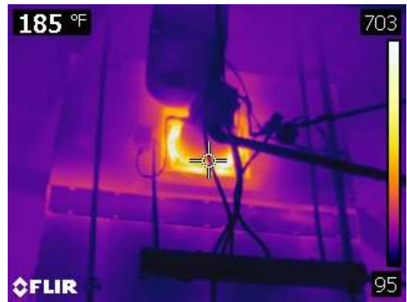
The main points of heat loss are on the back side of the ovens. Both upper and lower access points have high heat levels.
