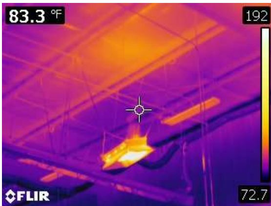
The heating unit above the foaming area is on and generating heat. There are a number of areas in the facilities that are being heated, but also have large air leaks to the outdoors.
